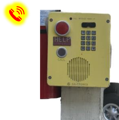
Emergency Call Box (Yellow Box)
